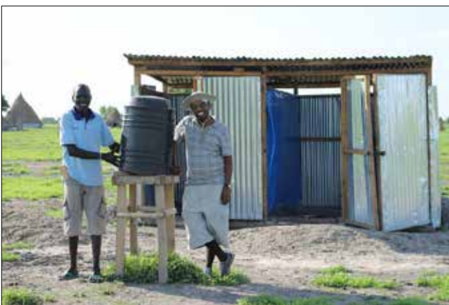
Fig 3. Community latrine construction in Mayendit, South Sudan. Photo by Amanda Patterson/Samaritan’s Purse
